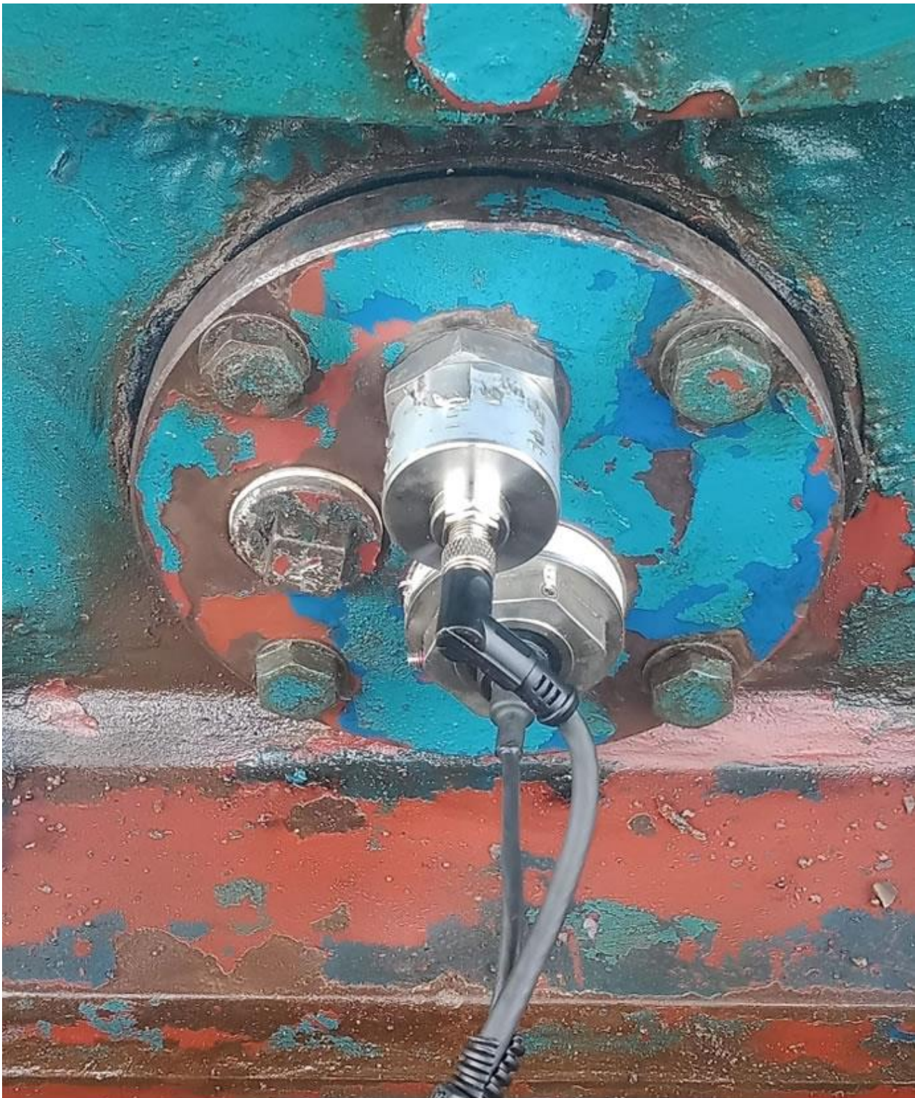
The sensor installed by Tehenomics on the mud pump.
