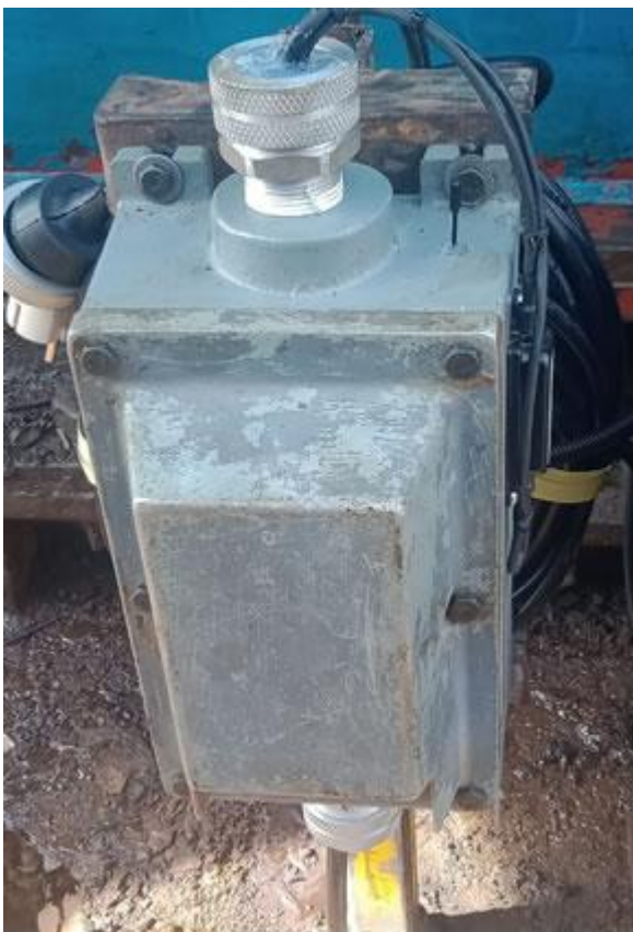
The Data Terminal Unit protected with an oil & gas standard enclosure
